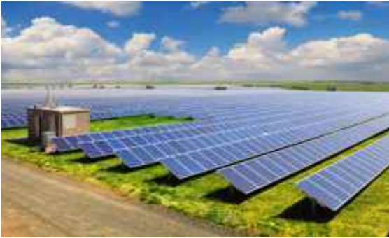
Photovoltaic Panel Solar Farm
