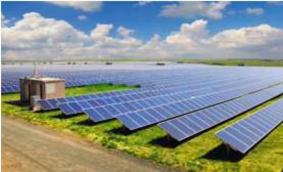
Photovoltaic Panel Solar Farm
